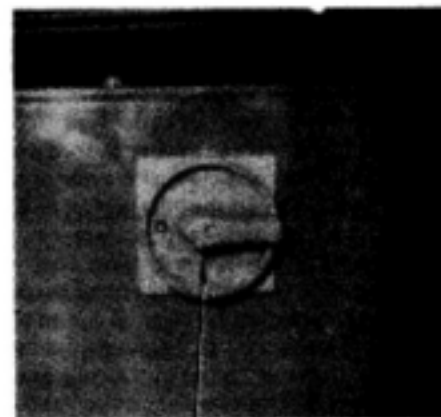
Isolator in OFF position
